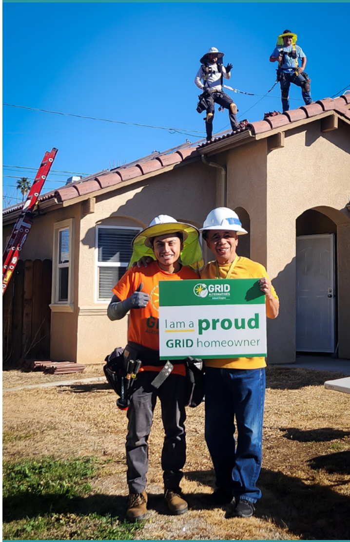
GRID IE's Daniel Montero , Solar Installation Supervisor, with Steven Chung homeowner. On the roof from GRID IE's Construction Team, Jeremiah Lee and Francisco PratsRamos
