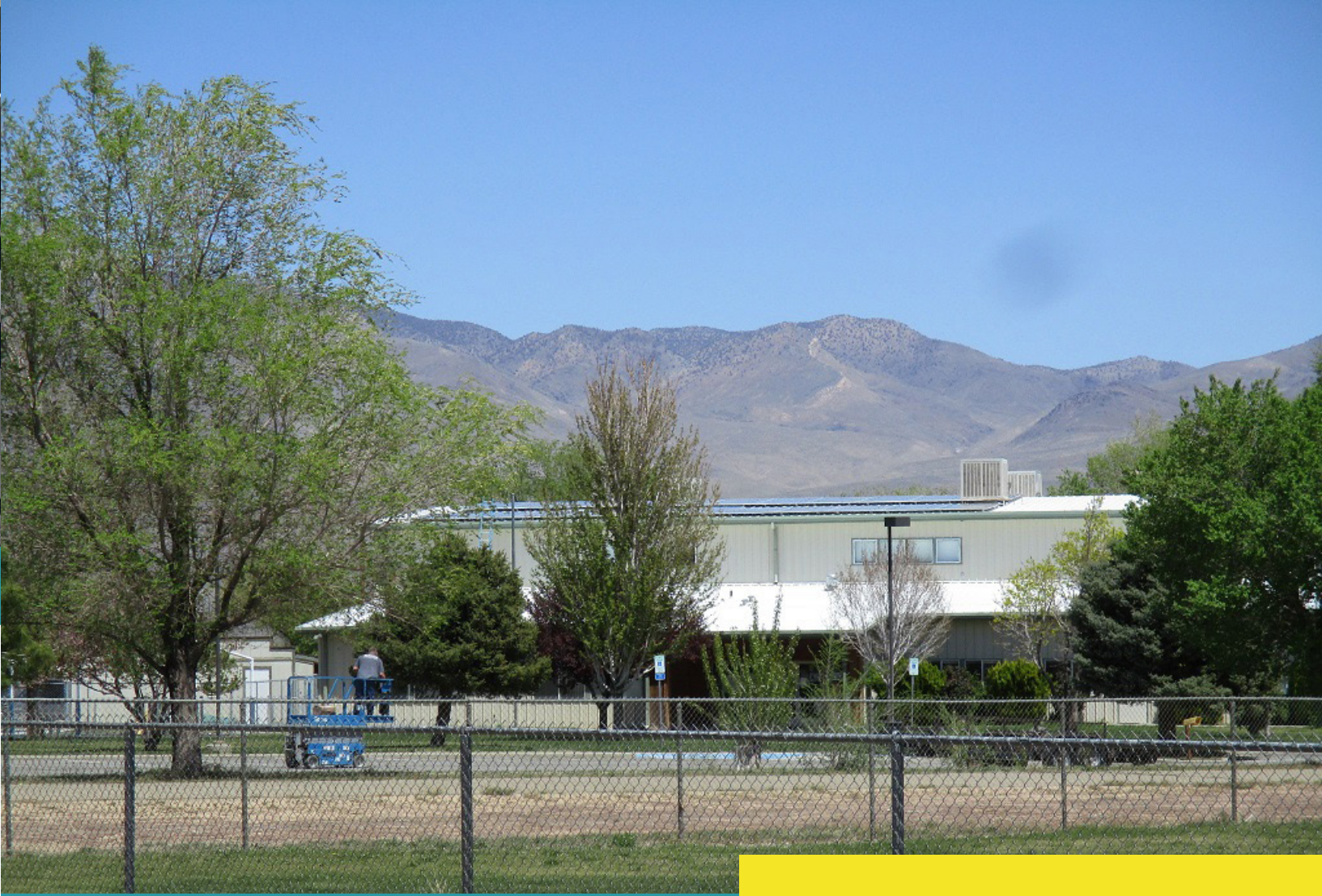
[ABOVE] Solar panels installed on the Alan Spoonhunter Memorial Gymnasium. [BELOW] Close up of the solar panels on the roof.
