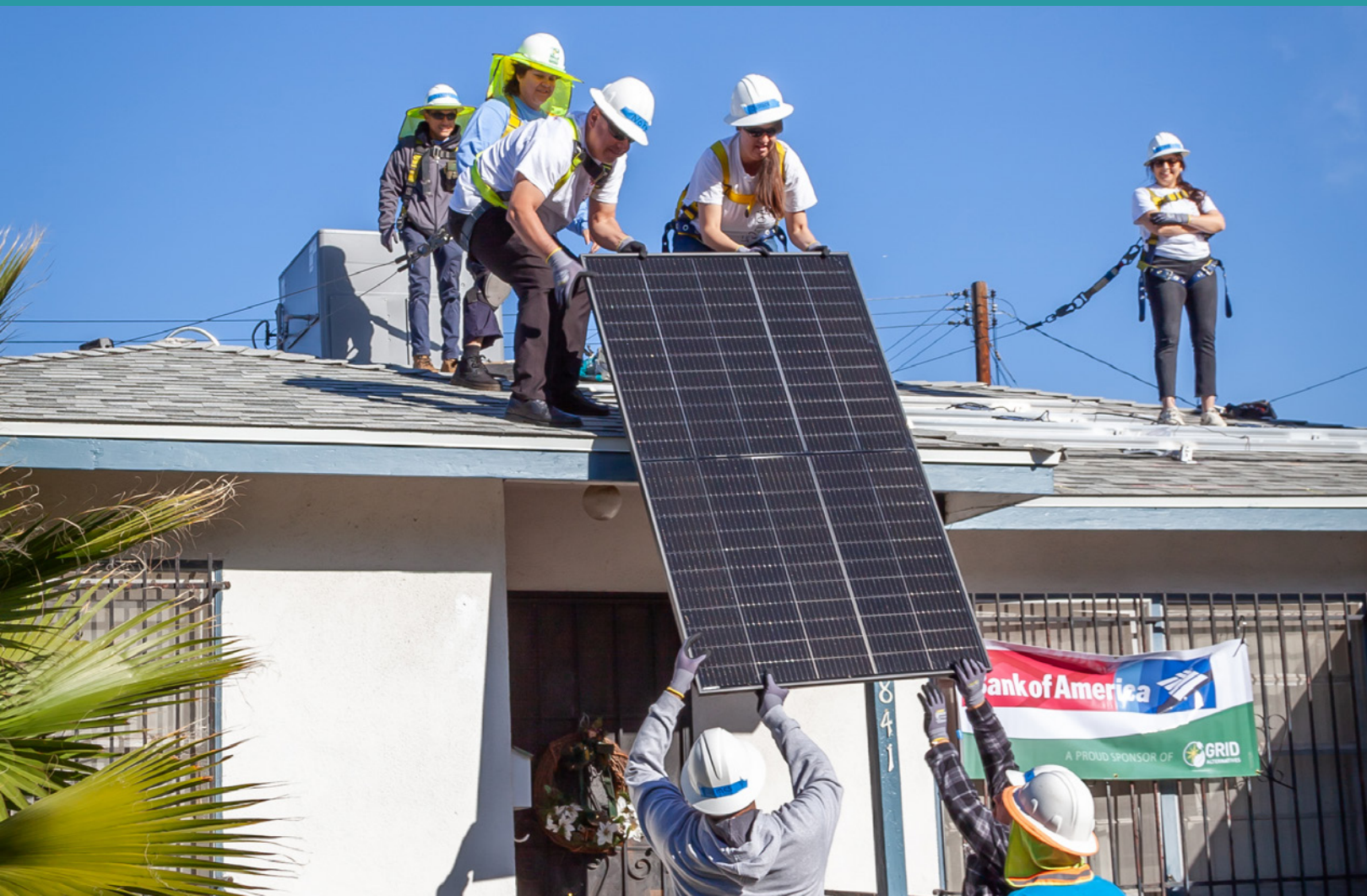
Bank of America volunteers installing solar panels on the roof of Rey’s home
