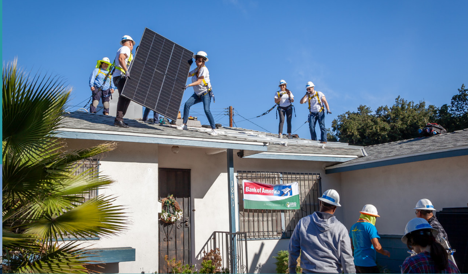
Bank of America volunteers installing solar in the Eastside neighborhood of Riverside, CA
