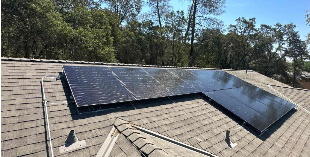
Figure 1. DAC-SASH funded solar PV array installed on a home in tribal land
