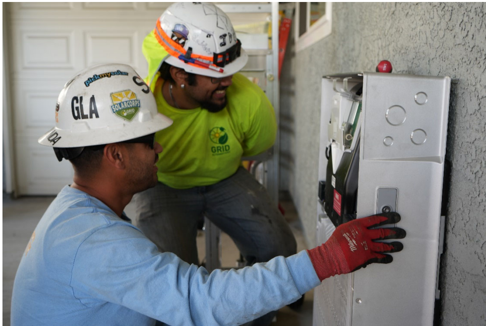
Figure 4. GRID staff inspecting a battery they just installed (November 2024)
