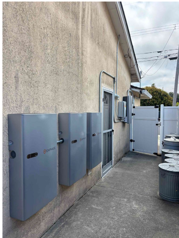
Figure 6. Enphase 5Ps installed (June 2025)
