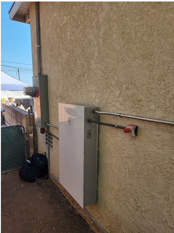
Figure 7. Tesla Powerwall 3 installed (September 2025)
