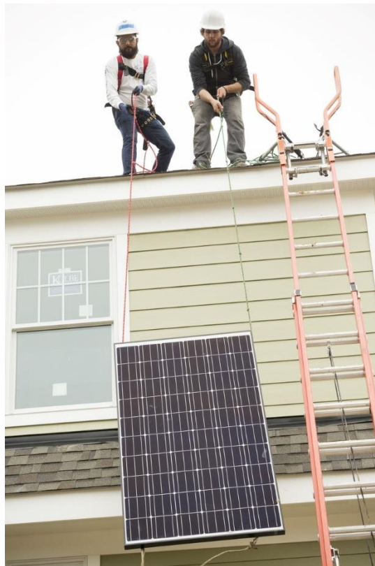
Volunteers with GRID Alternatives install solar panels on two homes Habitat for Humanity of Northern Virginia is building in Southeast Fairfax County. The two houses will be Habitat NOVA's first solar homes to receive solar panels and GRID's first solar installations in Virginia. (Photo credit: Mark Finkenstaedt for Habitat for Humanity of Northern Virginia).
