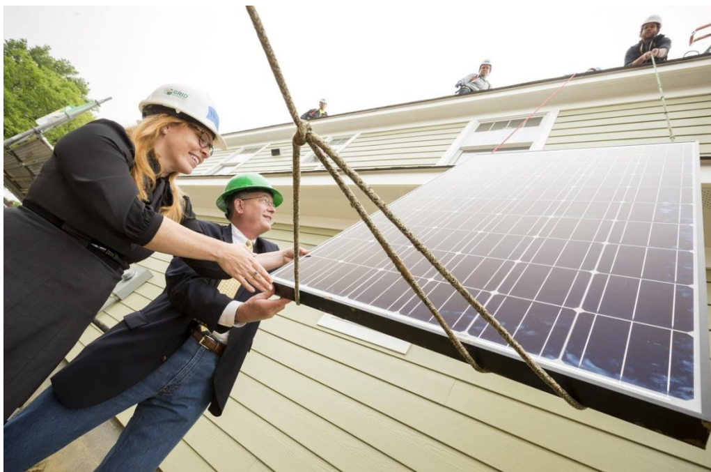
Jon Smoot, Executive Director of Habitat for Humanity of Northern Virginia, and Nicole Steele, Executive Director of GRID Alternatives, help raise solar panels to the roof of a new house Habitat for Humanity of Northern Virginia is building in Southeast Fairfax County. GRID Alternatives led the solar installation today – which marks the first Habitat NOVA homes to receive solar panels and GRID's first solar installations in Virginia. (Photo credit: Mark Finkenstaedt for Habitat for Humanity of Northern Virginia).
