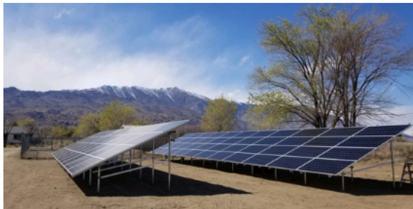
Solar now powers Big Pine Paiute's water well pump
